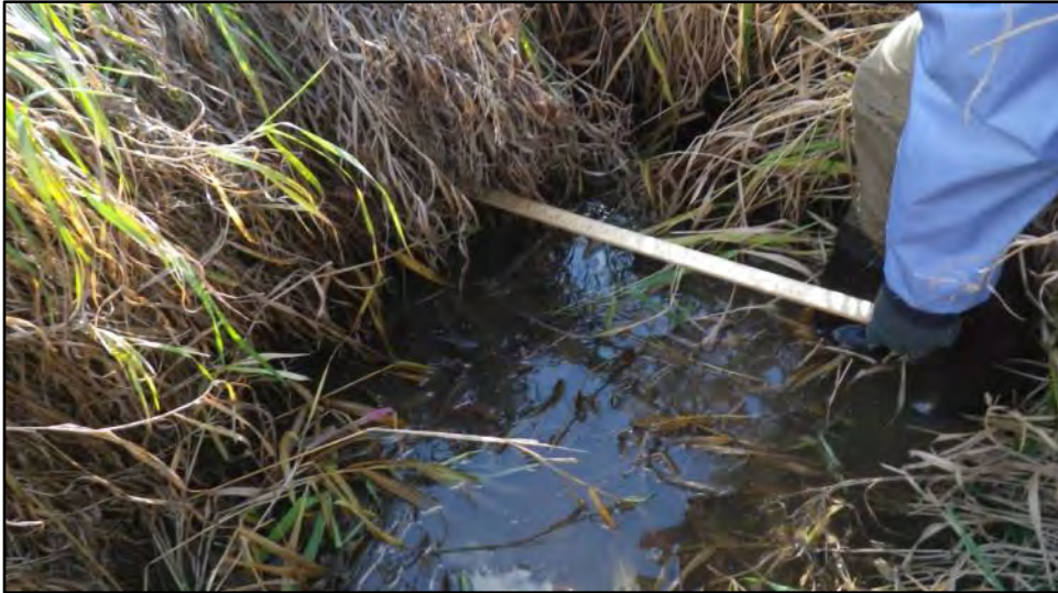
96. HT-2b-1 Severe undercutting found at parts of the reach. Up to 0.30m of undercutting observed.
