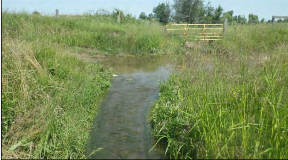
74. E-T1-1 Channel crossing farm lane with no CSP.
