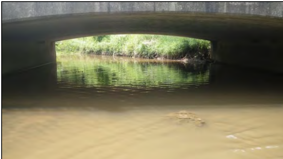
77. T1 Bridge crossing is quite low with major siltation underneath the structure.
