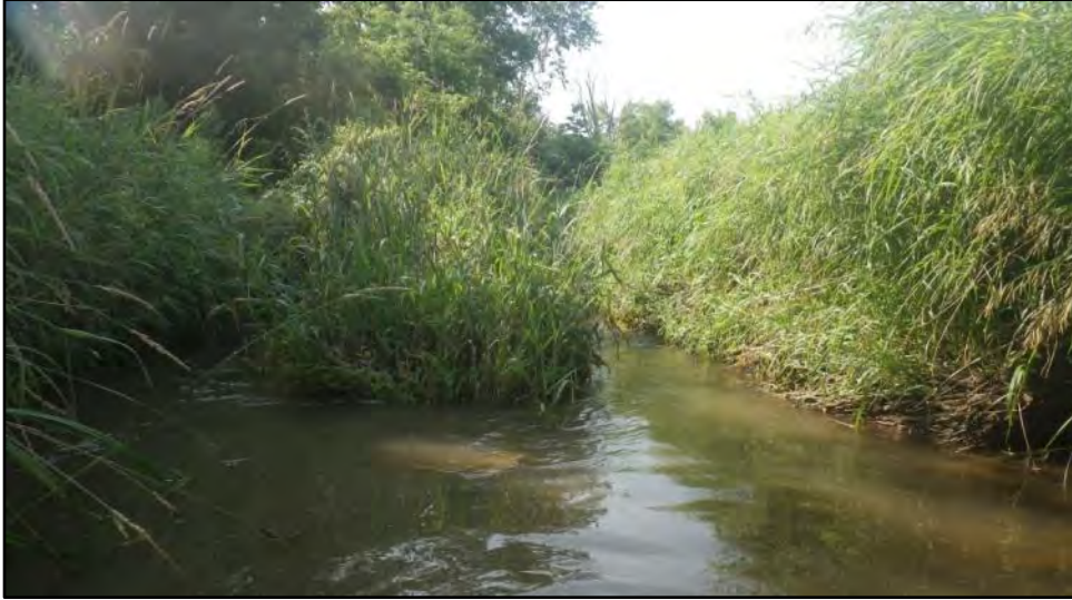
112. HT-1 Material that has slumped off bank has created island causing the flow to split.
