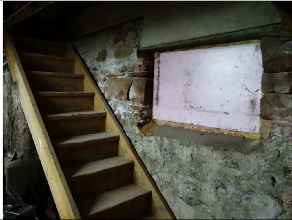
Plate 29: Detail of foundations, blocked windows, and un-used stairs in the basement at 94-96 Mill Street.
