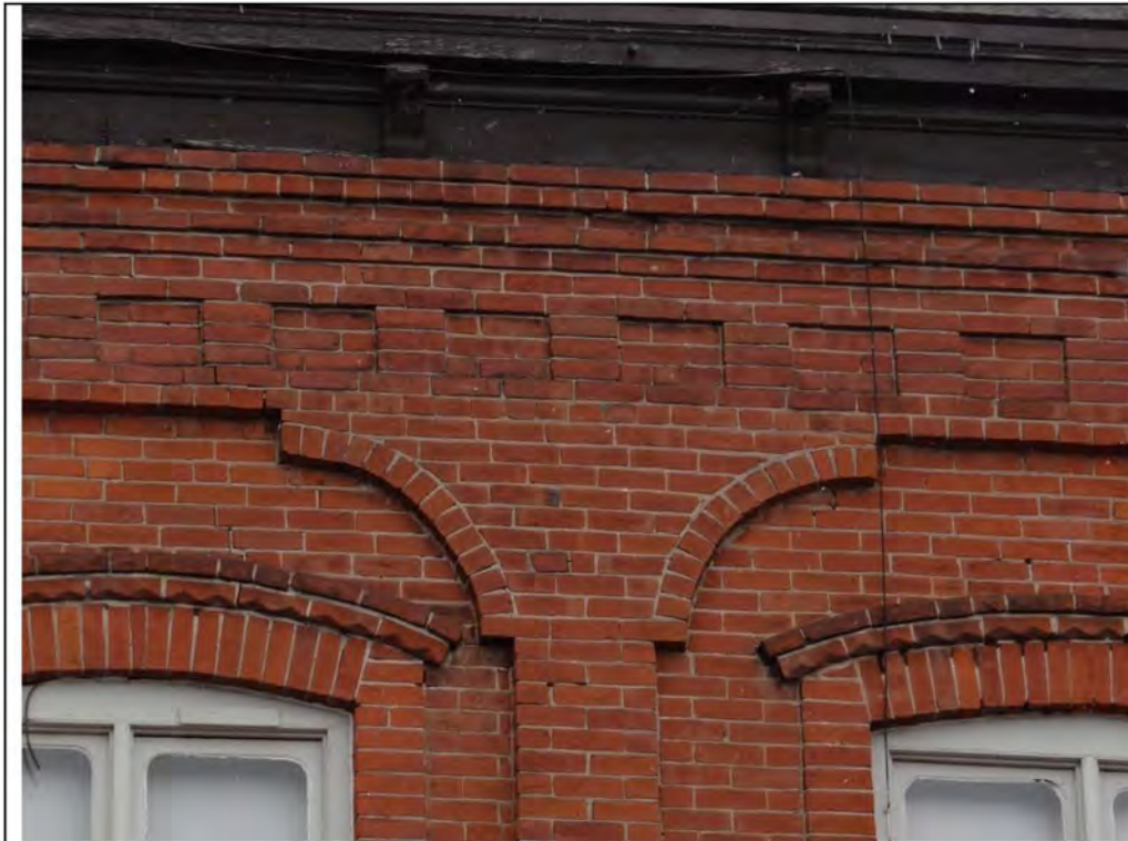
Plate 43: West elevation of 79 Main Street South, showing decorative brickwork, roof bracketing and segmental arches on the window, looking east.
