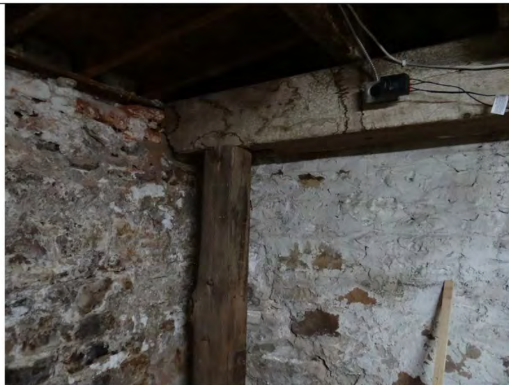
Plate 30: Detail of the foundation and large support beams in the basement at 94-96 Mill Street.
