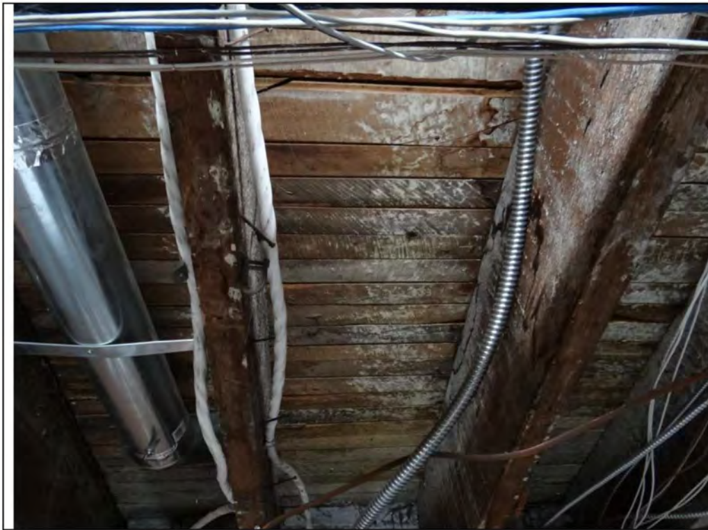
Plate 27: Detail of the sawn floor joists and softwood floor boards from the basement at 94-96 Mill Street.
