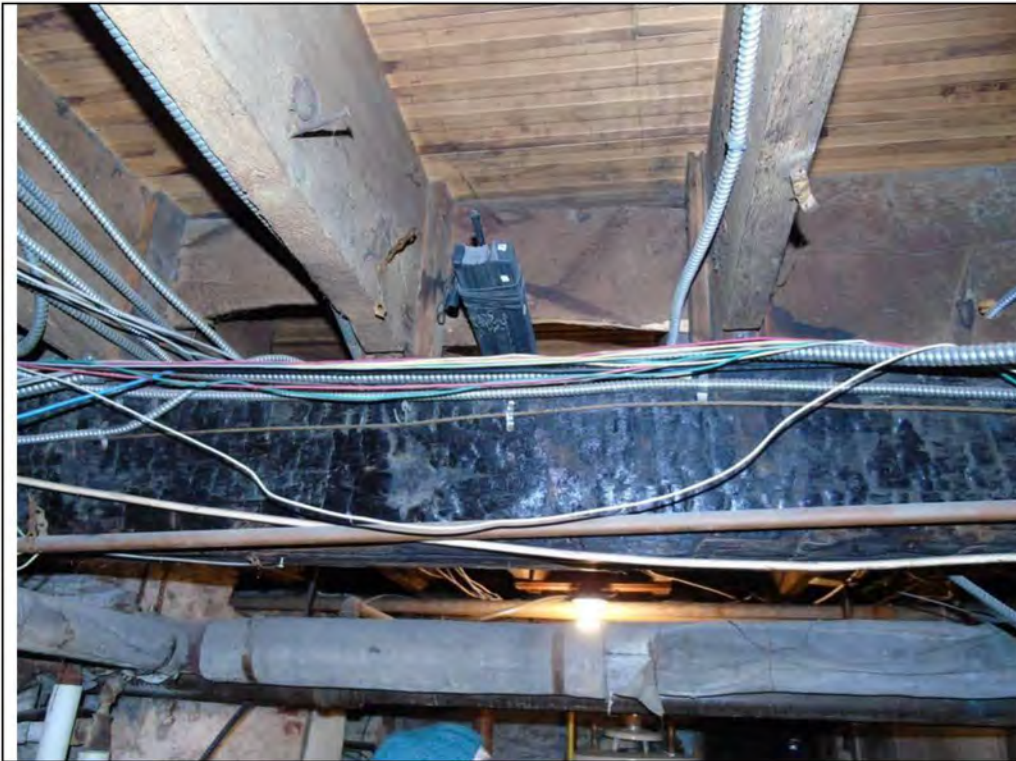
Plate 73: Basement of 79 Main Street South, showing charred hewn wooden support beam, damaged by 1880s hotel fire.
