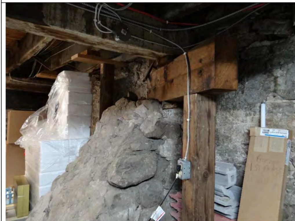
Plate 28: Detail of the stone buttressing and large support beams on the north wall of the basement at 94-96 Mill Street, looking northwest.
