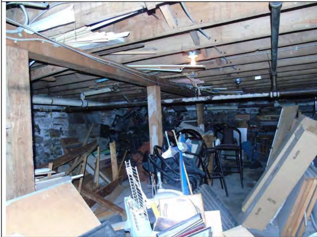
Plate 66: Basement of 71- 77 and 79 Main Street South, showing stone foundations, sawn beams, and modern dimensional lumber floor joists.
