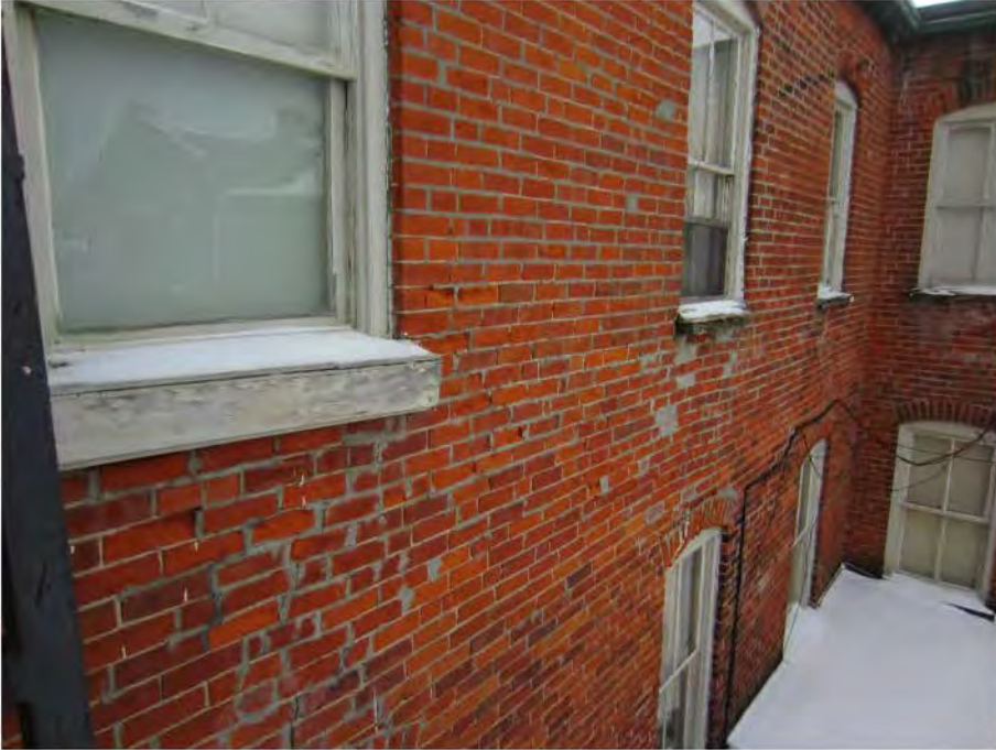
Photo #7: Visible cracks and repair on facade
