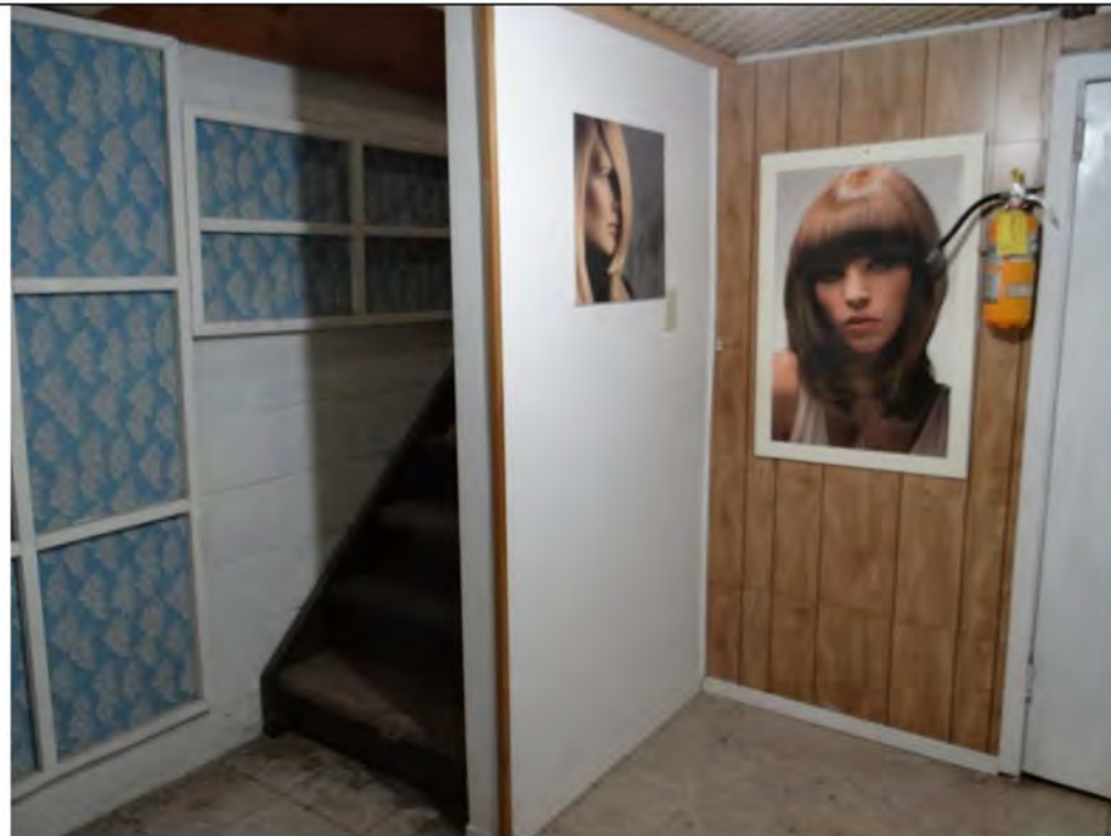
Plate 16: Detail of the finished section of the basement in the concrete block addition at 69 Main Street South.
