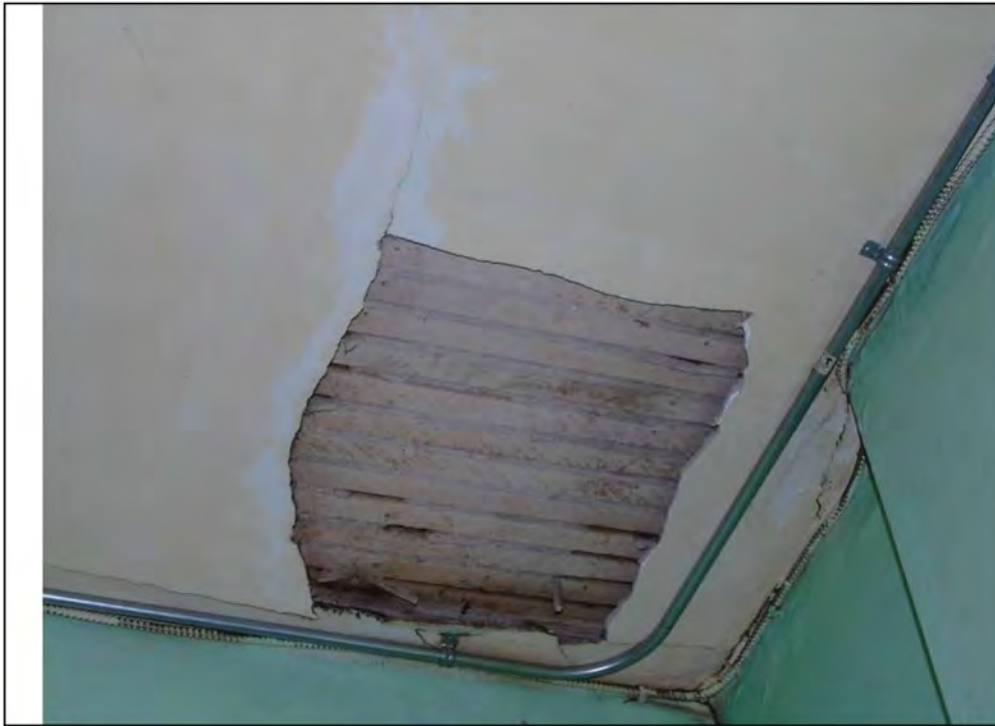
Plate 57: Original lathe-and-plaster was found throughout.
