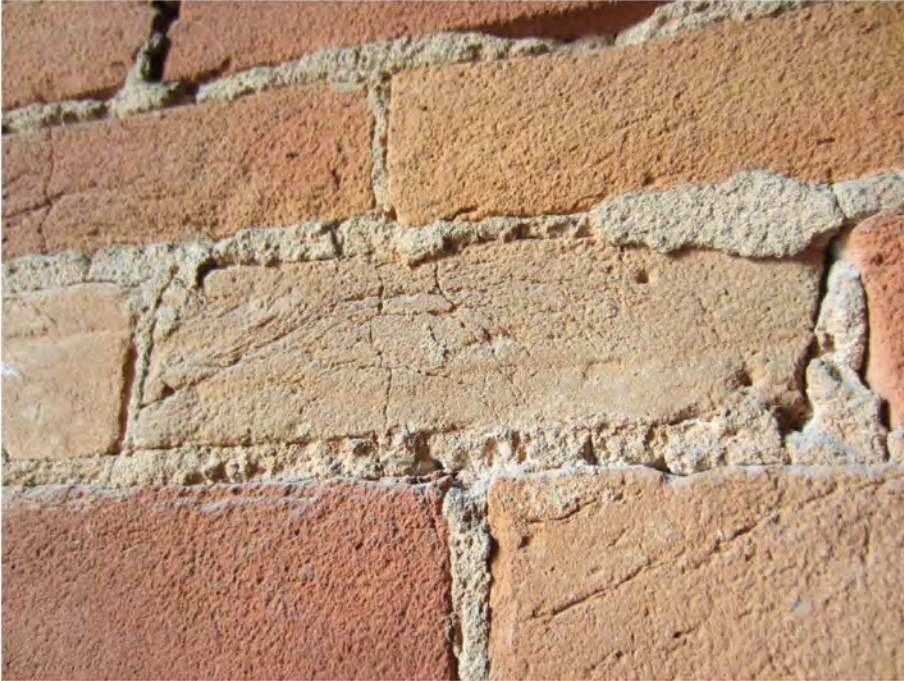
Photo #11: Visible cracks
