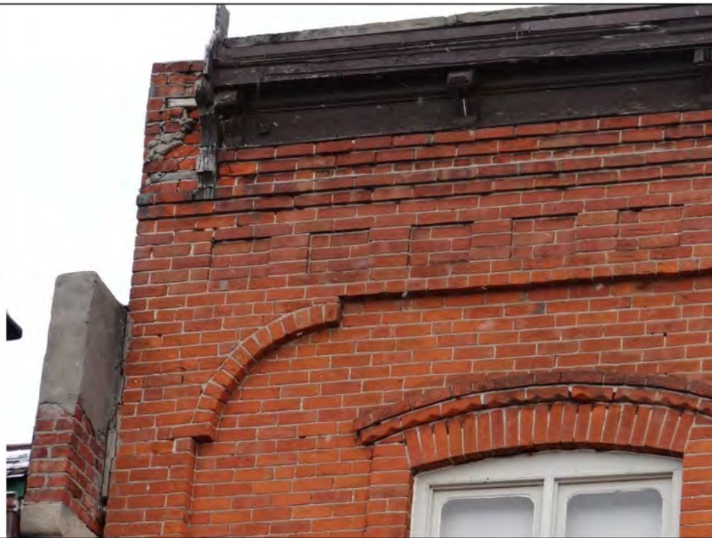
Plate 42: West elevation of 79 Main Street South, showing decorative brickwork, roof bracketing and segmental arches on the window, looking east.
