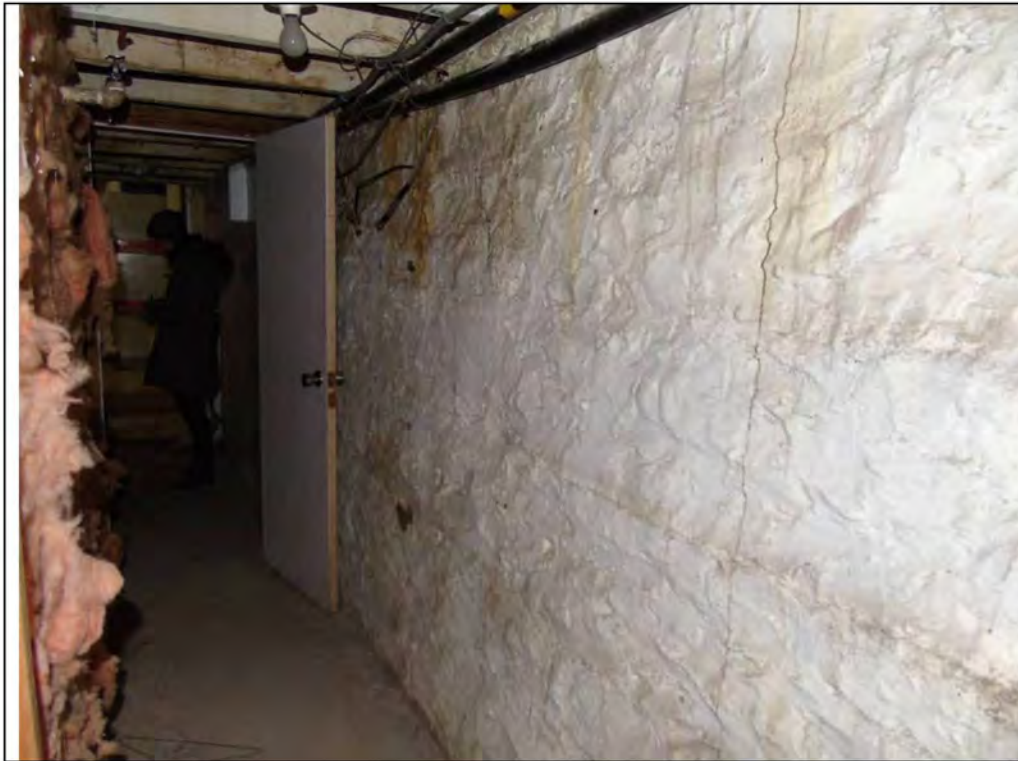
Plate 69: Basement of 71- 77 and 79 Main Street South, showing painted stone foundations at right, and modern insulated walls at left.
