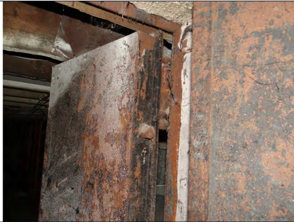
Plate 15: Detail of the Bank of Hamilton vault door in the basement of 69 Main Street South.
