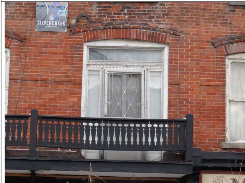
Plate 44: West elevation of 79 Main Street South, showing second floor doorway and balcony, looking east.
