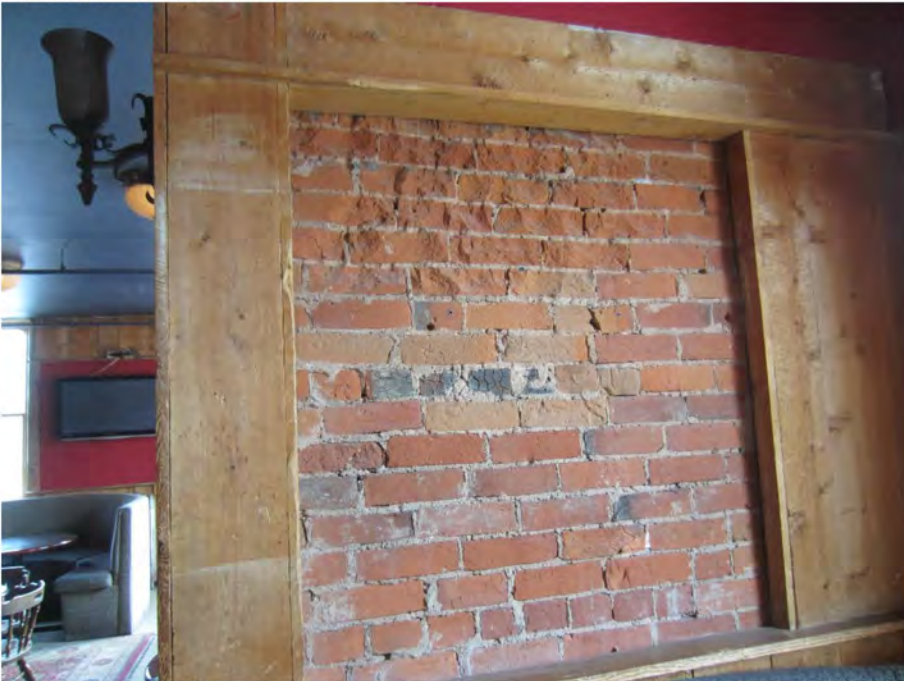
Photo #10: Visible cracks and spalling
