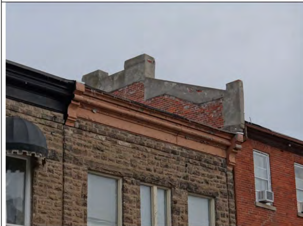
Plate 2: West elevation roof, cornice, and parapet of 69 Main Street South, looking southeast.
