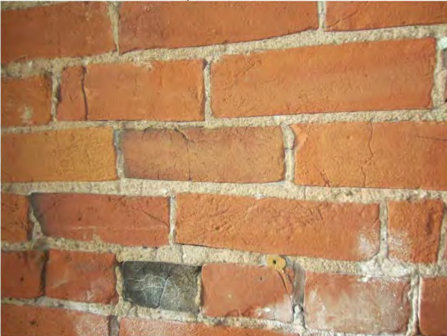
Photo #8: Visible cracks
