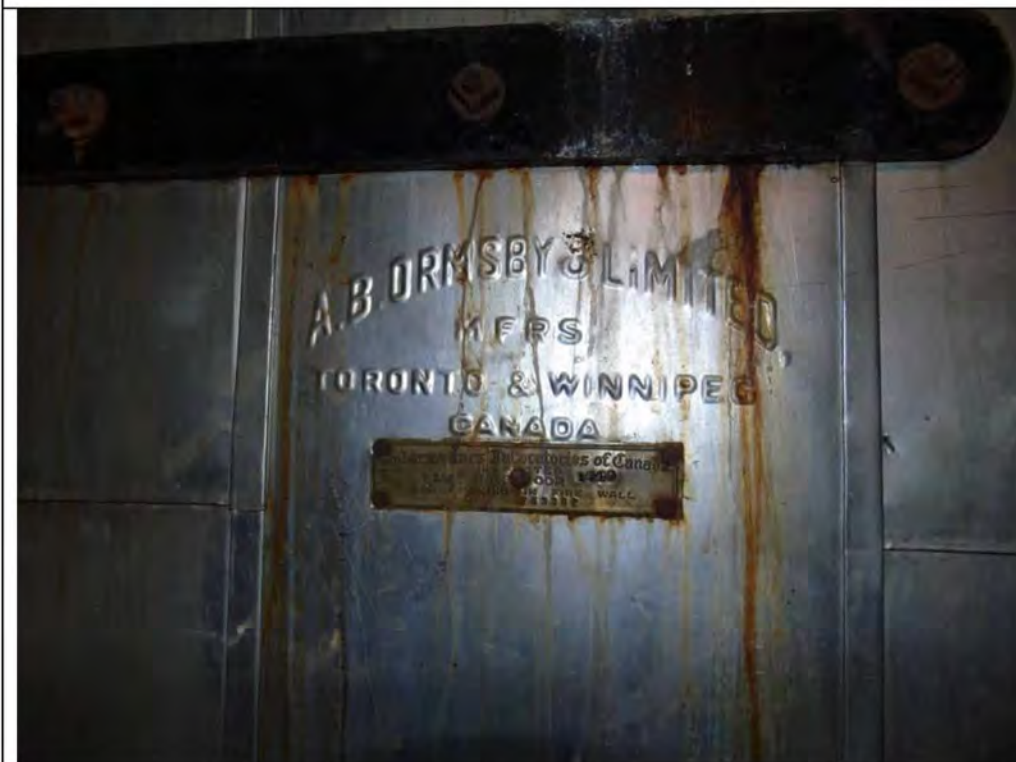
Plate 72: Basement of 71- 77 and 79 Main Street South, showing heavy metal boiler room door.
