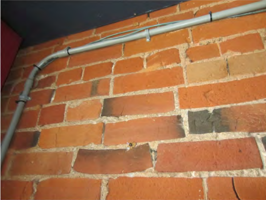
Photo #9: Visible cracks
