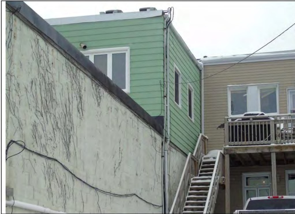
Plate 5: East elevation of the second floor of the modern rear addition at 69 Main Street South, looking southwest.
