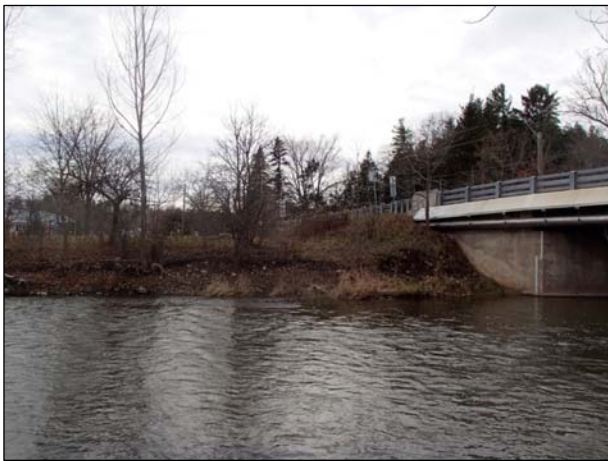
Photo 3: Right bank erosion downstream of bridge
